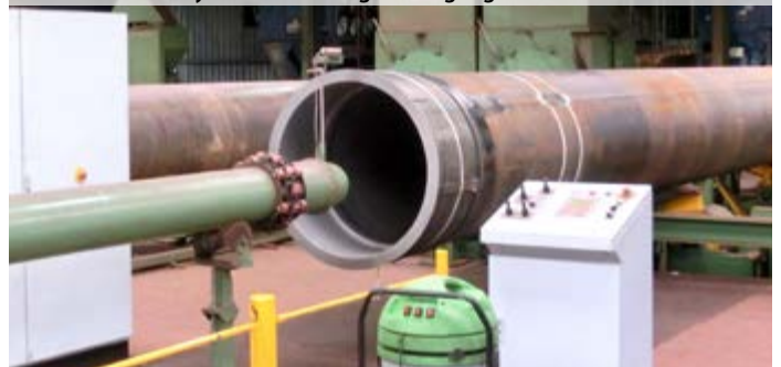
► Internal coating of cooling water intake risers for extensive FLNG-Project in Australia – only available in English language
